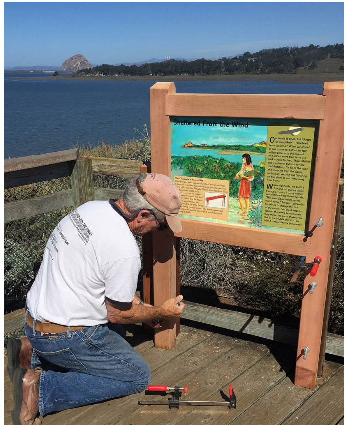
Craig Johnsen, who built the frames, completes installation of one of the new panels at Bush Lupine Point.
