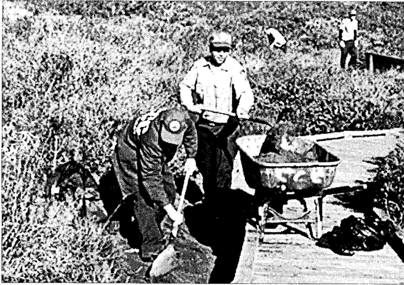
Four members of a CCC work crew that volunteered their time for four days in March, cleared away sand that had blown against the boardwalk, to prevent the timbers from rotting. Photo by Yolanda Waddell.
