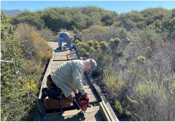
Team replacing damaged boards. Jeff Reifel in foreground. Photo by Jeff Reifel
